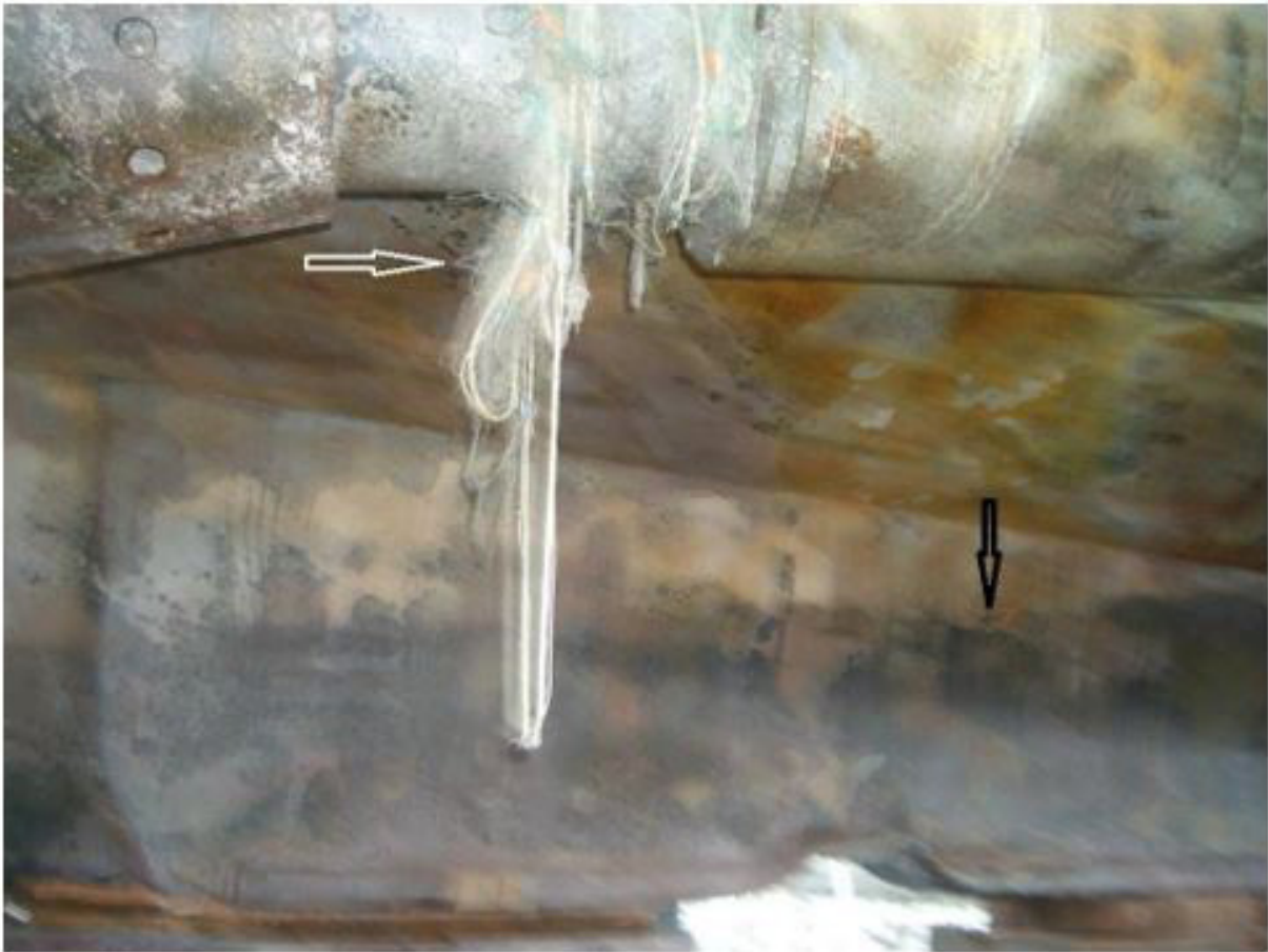
Figure 11: The tangled fishing net wires (white arrows) on the propeller axis indicate the running aground prior to the explosion and the black charred hull surface (soot) may be due to the flame at the moment of the blast for an underwater explosion (black arrows). Also, it cannot be ruled out that the strong ICCP current might flow on the hull surface when it ran aground before the underwater explosion [3,7]
